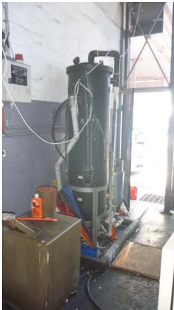
Photo 4: Oil separator at covered mechanic workshop area at 650-658 Canterbury Rd
