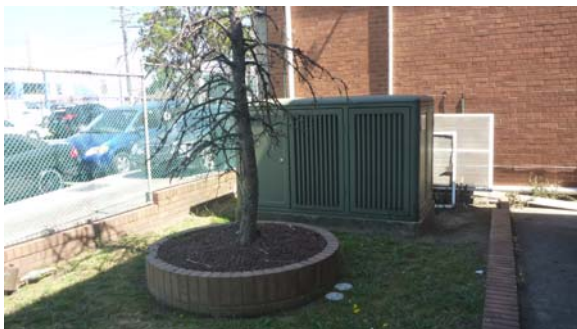
Photo 8: Electrical sub-station located at the north-western corner of 2B, 2C-2D Liberty St (looking north)
