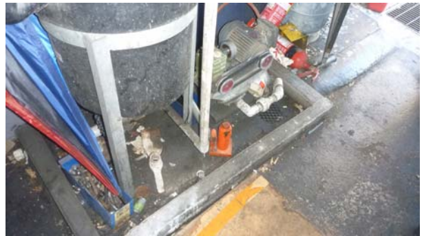
Photo 5: Oil separator at covered mechanic workshop area at 650-658 Canterbury Rd
