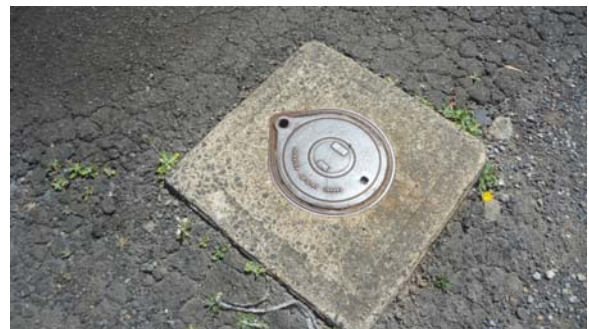
Photo 9: UST filling point located south of the south-western building corner at 2B, 2C-2D Liberty St (looking north)
