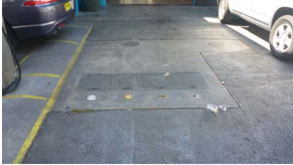
Photo 1: UST filling points at former service station at 650-658 Canterbury Rd, (looking south-east)
