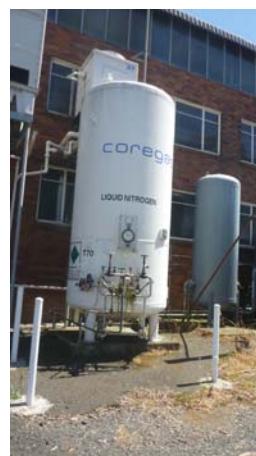
Photo 11: Liquid nitrogen AST at 2B, 2C-2D Liberty St (looking north)
