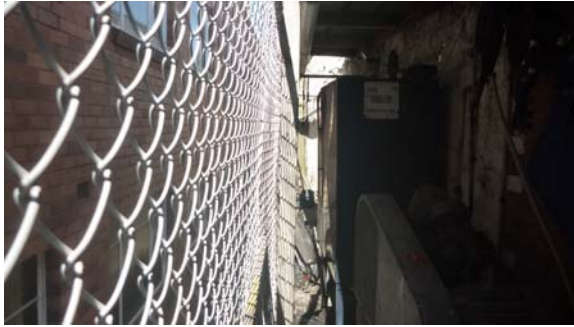
Photo 6: Oil AST rear of covered workshop at 650-658 Canterbury Rd (outside the southern office wall – looking south-west)
